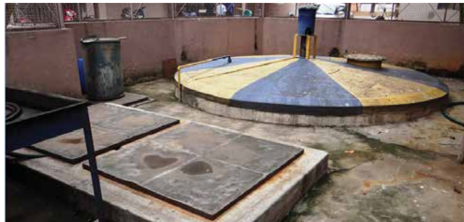
Sewage treatment plant (above); waste management (right); R.O. water system (below right); rain water harvesting (below) at KSCA's M. Chinnaswamy Stadium.
